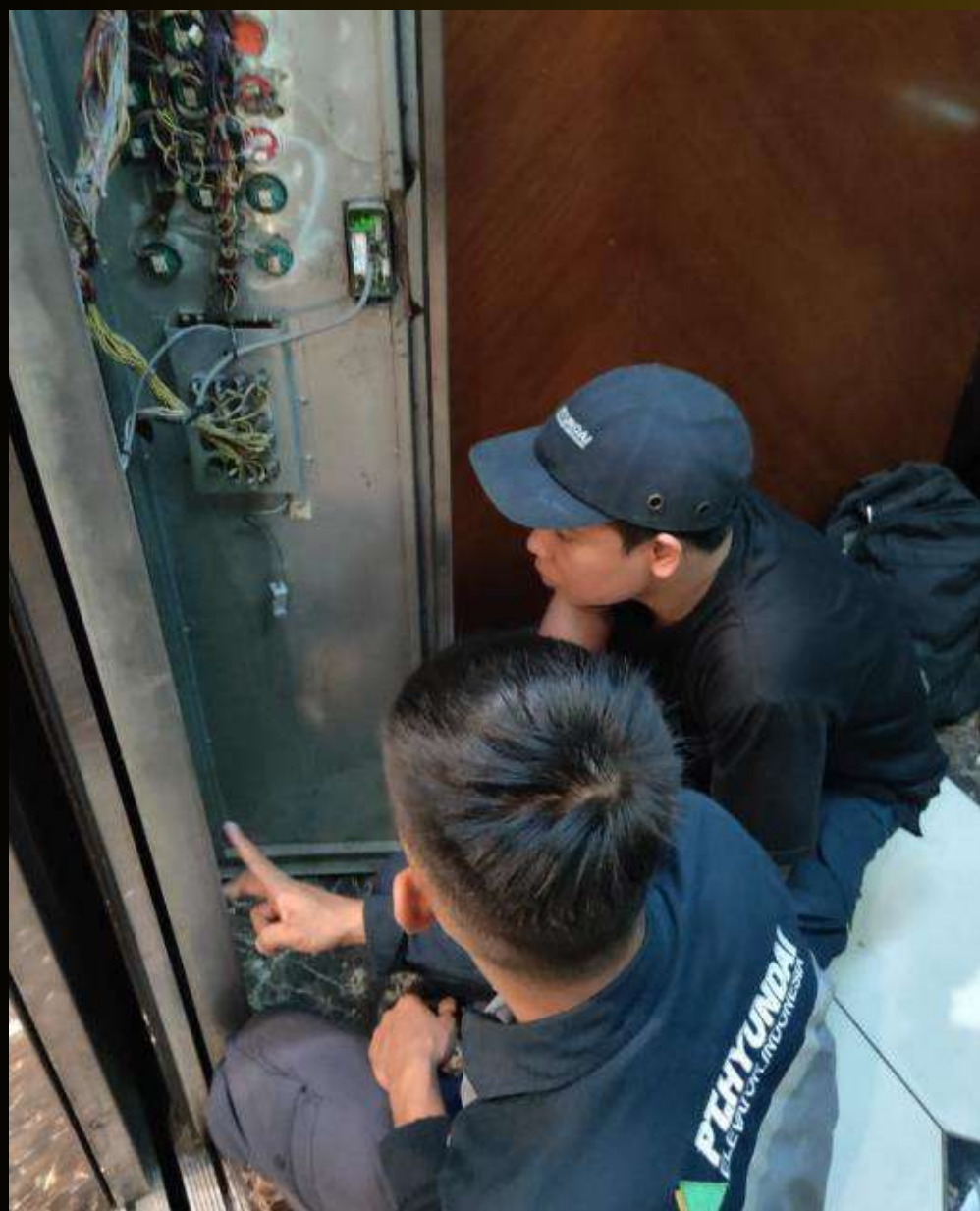
PERGANTIAN INTERCOM LIFT
